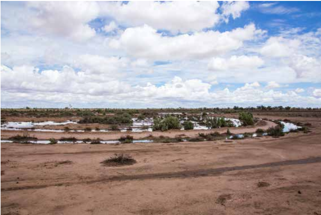
Figure 8: Waterpond established in 2012. From the foreground: scalded area, external borrow trench, pond wall, inner borrow trench, reclaimed area. The water is from 30 mm of rainfall in an overnight storm.
